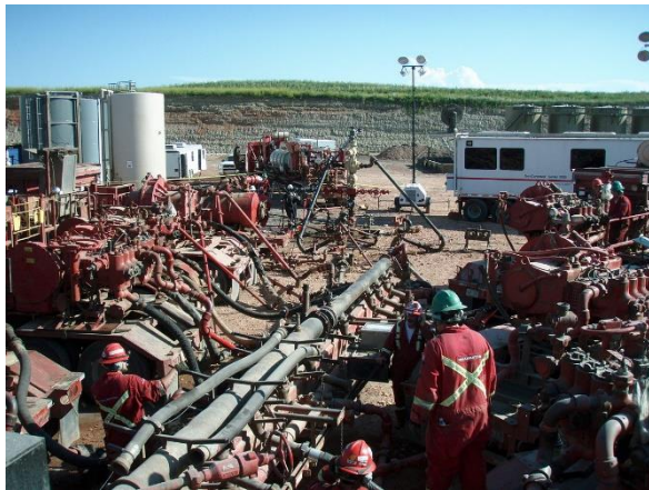
Figure 3 Typical piping and pad site setup
