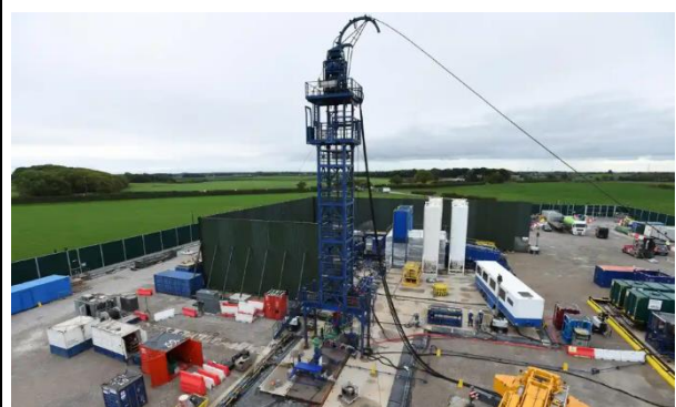
Figure 2 Typical Fracking Rig
